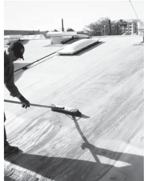
First, clean the roof thoroughly with TSP or TSP substitute, push broom, and water.
