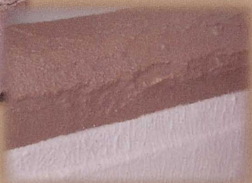
Parapet patched with Duratex Stucco ↔
