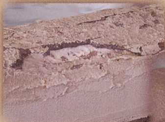
↔ Roof parapet in need of repair
