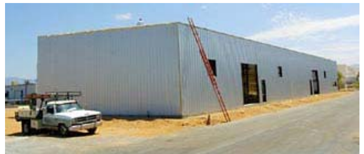
Construction continues on a new storage facility for Elastek, 3700 S. Palo Verde Road.
